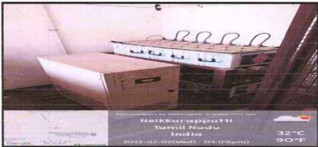
Admin Block – UPS Room
